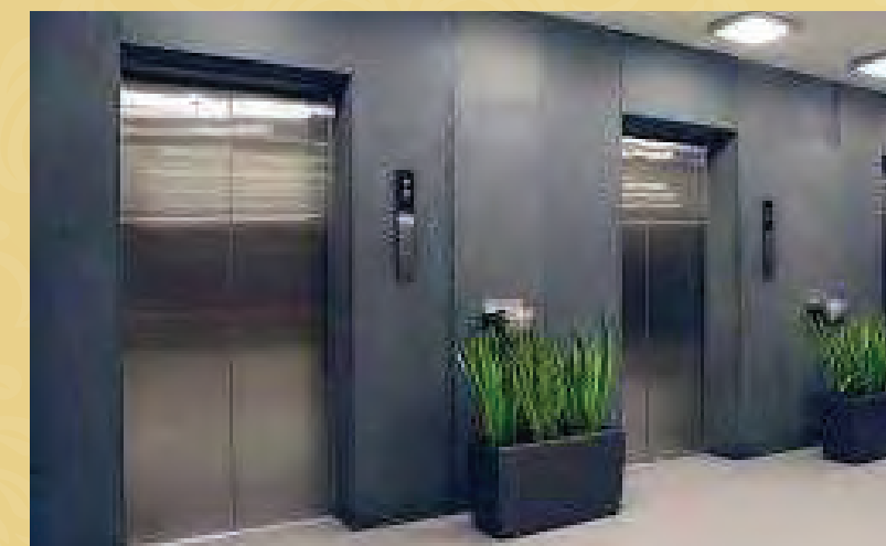
2 HIGH SPEED LIFTS IN EACH WING
